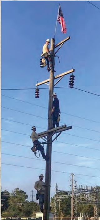
In a sign of recovery from Hurricane Ida, Tishomingo County crew members replace an American flag hanging over Washington-St. Tammany Electric's Slidell yard. PHOTO BY DANNY WOOD
