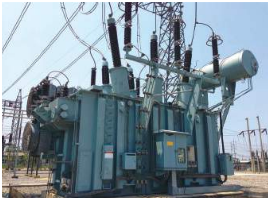
Transformers are a hot commodity for electric utilities. Steel shortages, coupled with a lack of manufacturing workers, mean transformer manufacturers are unable to keep pace with a significant increase in demand. ADOBE STOCK PHOTO BY CHII CHOBITS
